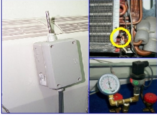
Fig.6 Evaporator and the transducers
