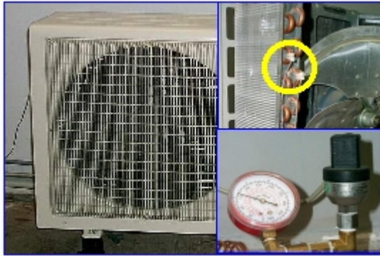
Fig.7 Condenser and the transducers
