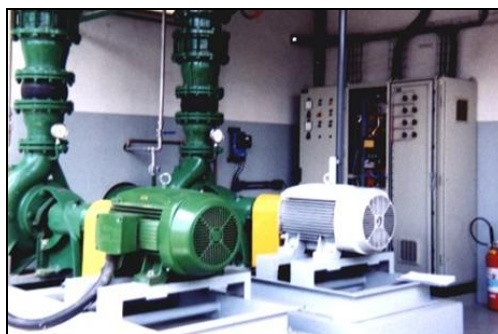
Fig. 10. Identical drives with motors of rated power of 100 hp, standard and high-efficiency types.
