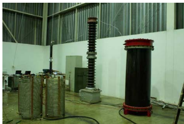
Fig. 22 – Calibration test setup at the lab – step-up transformer (at right), CVT (center), CVD (at left) and 1mH inductances used for reactive compensation (front).
