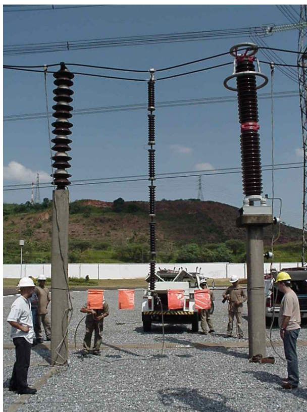
Fig. 1 – Capacitive voltage divider (CVD) – installation for measurements in a 345kV substation.
