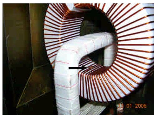
Fig. 2 VL on the low-voltage side of CRCT
