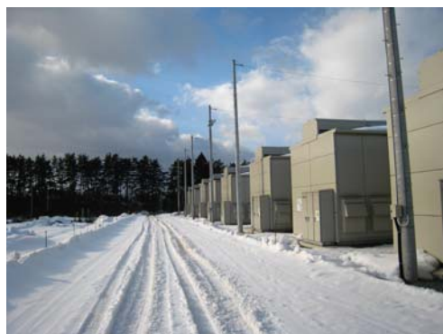
Fig.19 NAS battery systems in wind-farm
