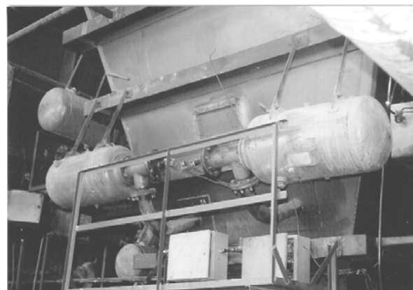
Fig. 3. Large capacity ABD mounted on the metallic wall of bunker for coal storage in large electro-thermal plants
