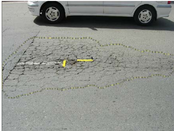
Fig.1. Digital measurement of an alligator cracking.
