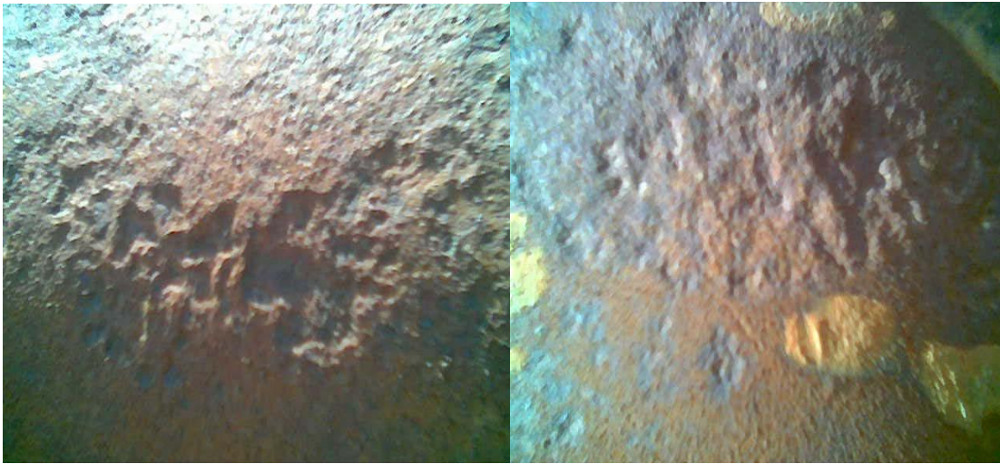
Figure ۱.۴- corrosion under insulation in maroon desalting plants
