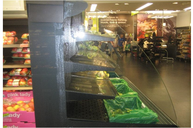
Fig.3 Upper shelf of a display cabinet extended causing the loss of the air curtain.
