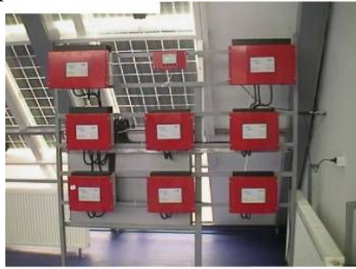
Figure 5. The inverters and Sunny Boy Controller
