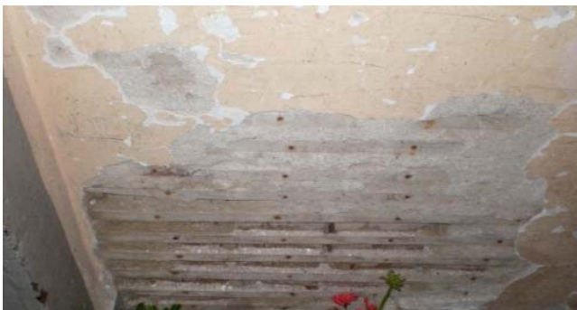
Fig.9 - Conservation state: Deteriorated
