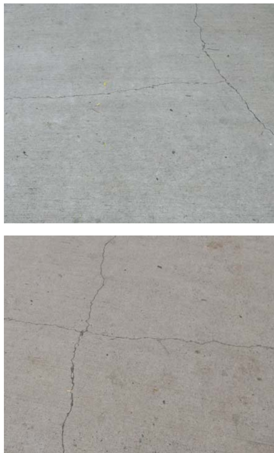
Figure 3. Transverse cracks due to restrained shrinkage
