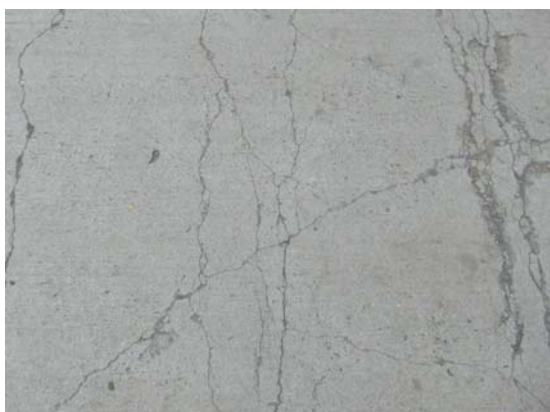
Figure 6. Closely spaced cracks parallel to transverse and longitudinal joints
