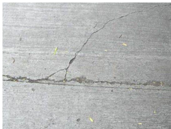
Figure 7. Saw-cut construction joints were not deep enough, so cracking of concrete occurred in the vicinity
