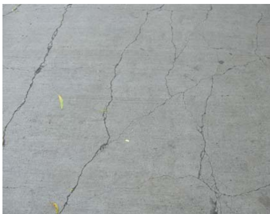
Figure 4. A network of fine fissures on the concrete surface
