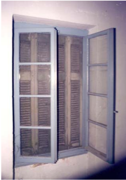
Fig.16 Venetian blinds direct the incoming air.
