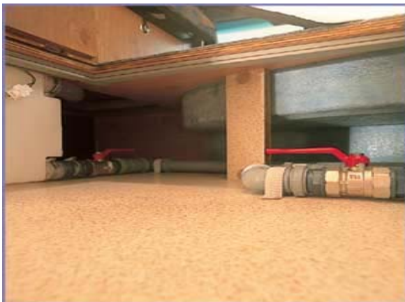
Fig. 8 Water tank and piping in the double pavement.
