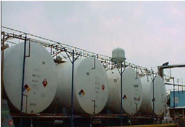
Fig. 1 Horizontal cylindrical tanks from the Company Sherwin Williams. S. A. de C. V.
