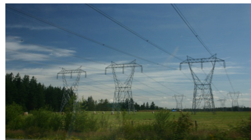
Fig 4 Transmission Line Towers
