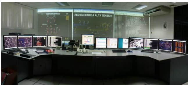
Fig. 5. On-Line Simulator installer at Distribution Control Center of Tampico Zone.
