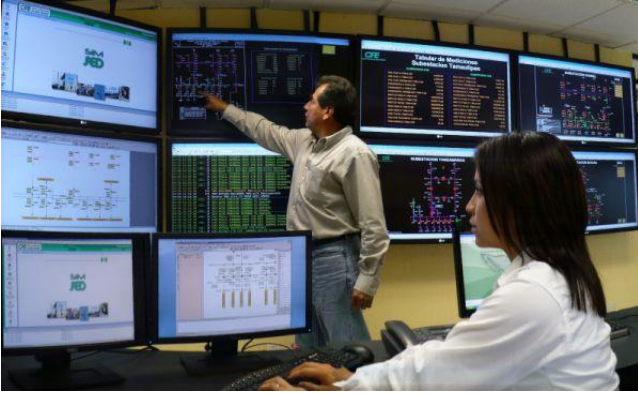
Fig. 6. On-Line Simulator installed in Monitoring and Analysis Center at Division Golfo Centro.
