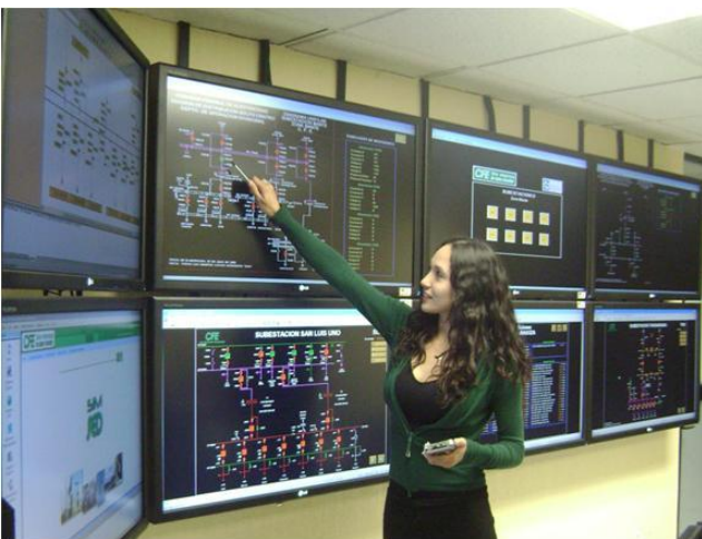
Fig. 7. Monitoring and Analysis Center for Regional Operators and analysts at Division Golfo Centro.
