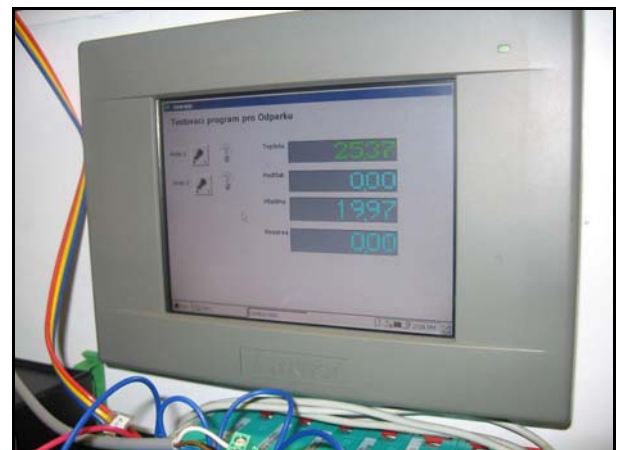
Fig. 10 Main window of a test program running on the TPC-650 panel PC.
