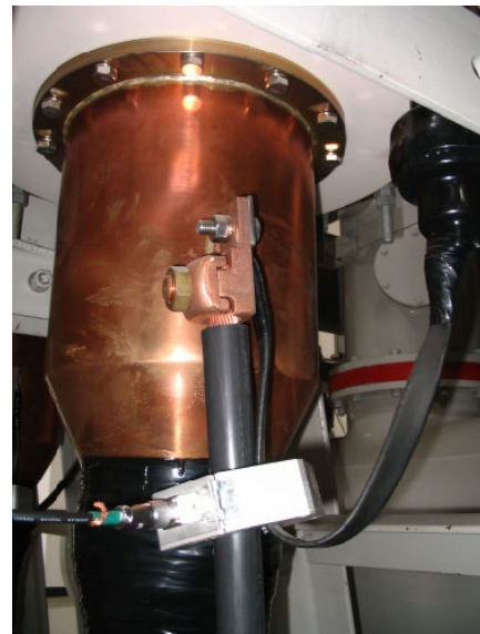
Fig. 2 HFCT installed around the earthing strap of cable termination.
