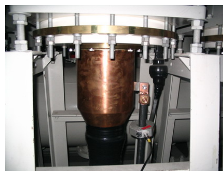
Fig. 2 HFCT installed around the earthing strap of cable termination.
