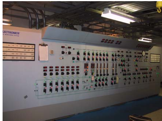
Fig.2 Typical status and control panel for an ARTCC site. (Courtesy of the FAA)
