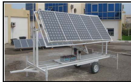
Figure 3: Photo of the solar refuel station
