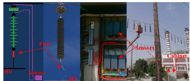
Fig. 6. A drawing of the basic leakage current measuring installation and photos from the actual installation in TALOS High Voltage Test Station
