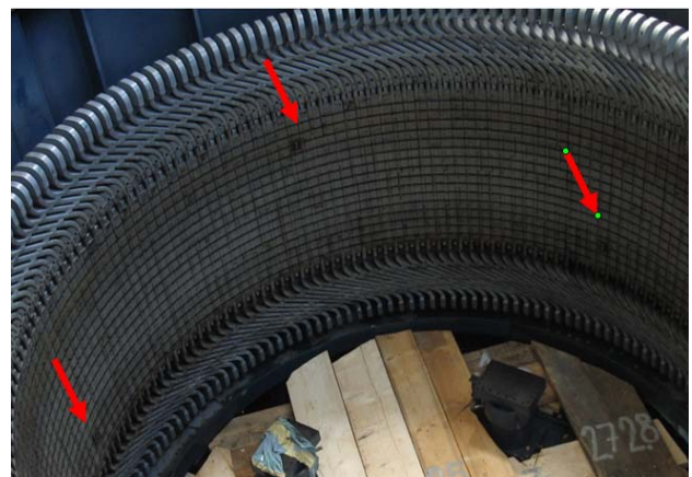
Fig.2 Detail of installed flux probes
