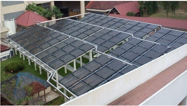
Figure 4: installed evacuated solar collectors at HUKM hospital
