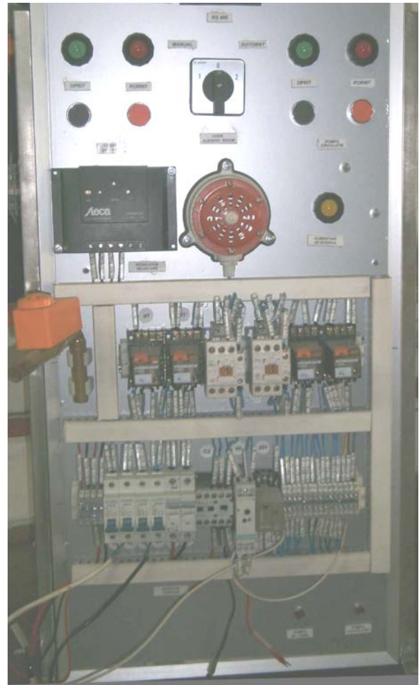
Fig. 3 Heating station control panel
