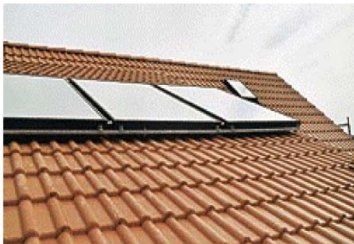
Fig.1 Disposition of solar panels
