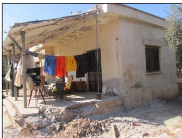
Figure 5: low quality of houses in Maras area
