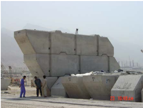
Fig.3 Precast sloping blocks for construction of block work quay wall, Pars Petrochemical port
