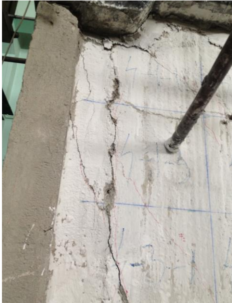
Fig.11 Diagonal crack that lead to failure
