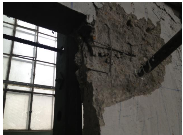
Fig.10 Right corner of the opening failure detail
