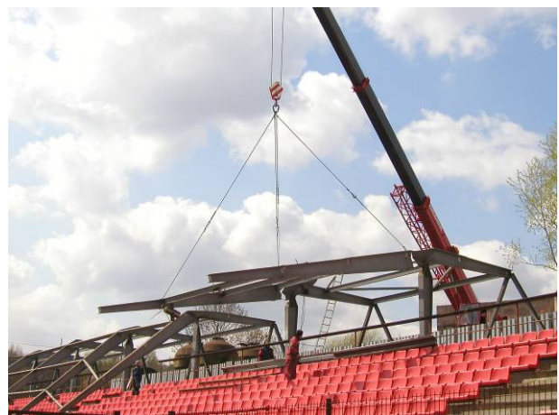
Fig. 2 View of the collapsed structure after dismantling of the coverings
