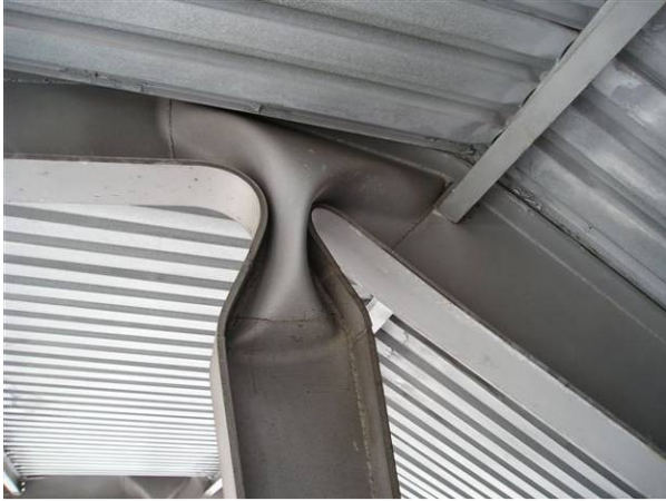
Fig. 3 Detail of the damaged joint in the part of structure with covering
