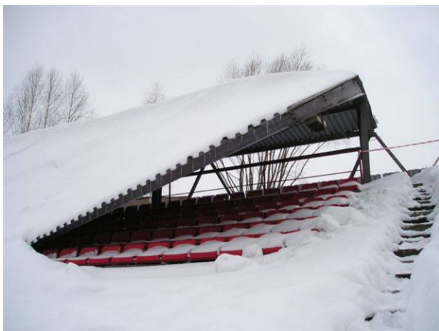
Fig. 1 View of the collapsed roof of the football stadium
