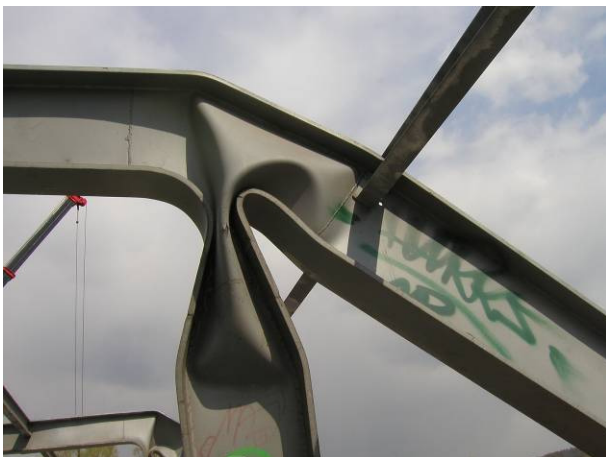
Fig. 4 Detail of the damaged joint in the part of structure without covering
