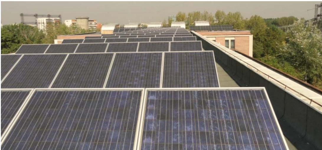
Fig. 1. University Politehnica of Bucharest, Faculty of Electrical Engineering Power Plant.
