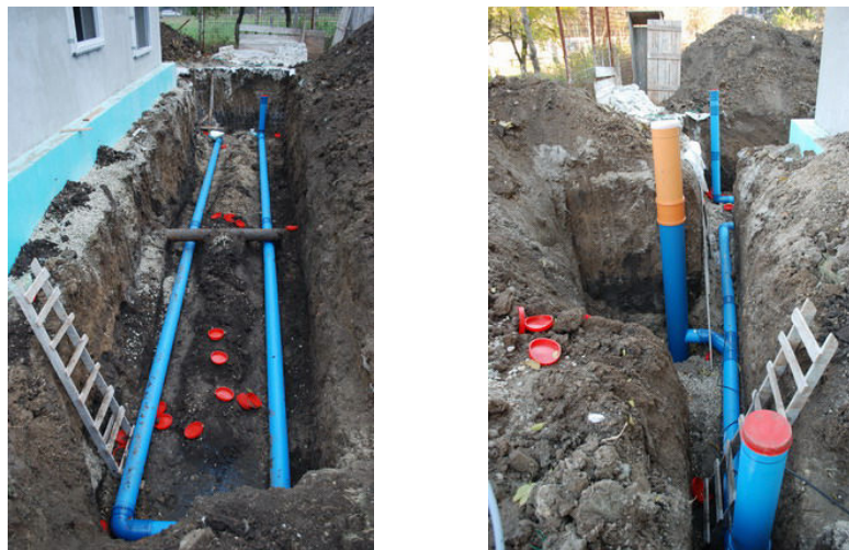
Fig. 8: Installation of the EAHX tube a) main side with fresh air intake; b) short side with condensation drain and house connection
