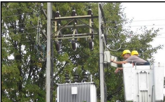
Figure 1. MIS-4S installed on pole TS 20/0.4 kV for checking the quality of power supply voltage
