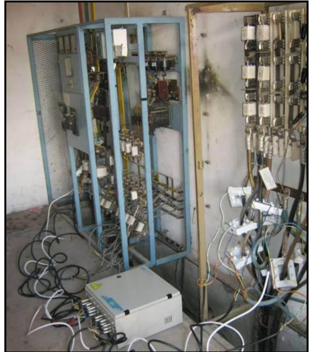
Figure 3. MIS-8 installed in TS 10/0.4 kV for closer localization of loss sources in the LV network
