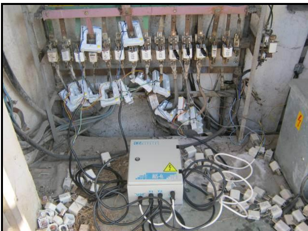
Figure 2. MIS-4S installed in TS 10/0.4 kV due to frequent overloads
