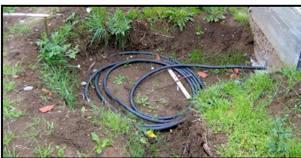
Figure 6. Problematic cable used for temporary connection of a site
