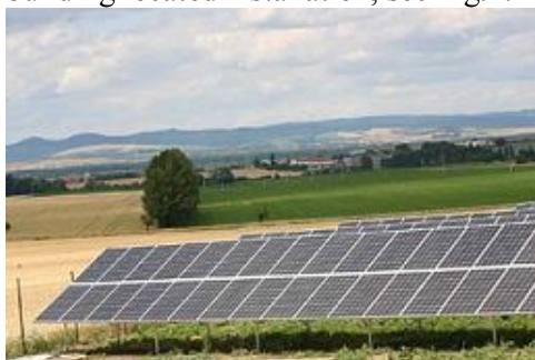
Fig. 3 Open field installation [2]
