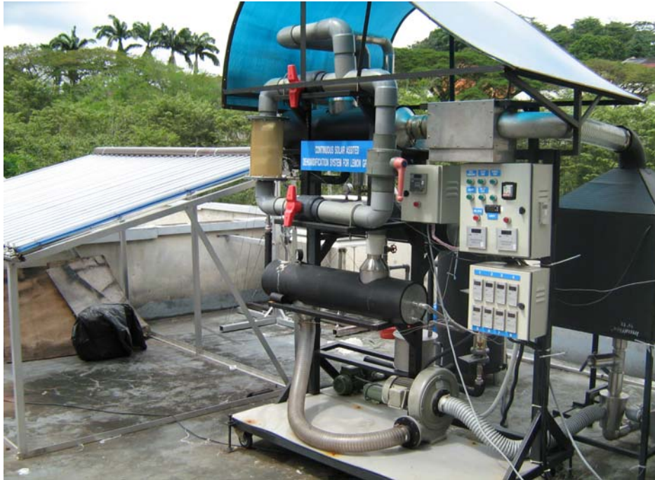
Fig.2 Photograph of the experimental set-up used, and for measurement of pressure at different locations of the system pressure gauges are used.
