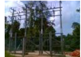
Step-up tx (0.45/11)KV
