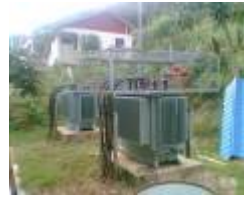
Step-down tx (11/0.45)KV
