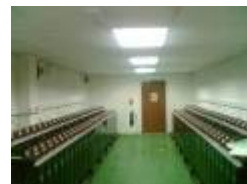
480KWh Battery Banks
