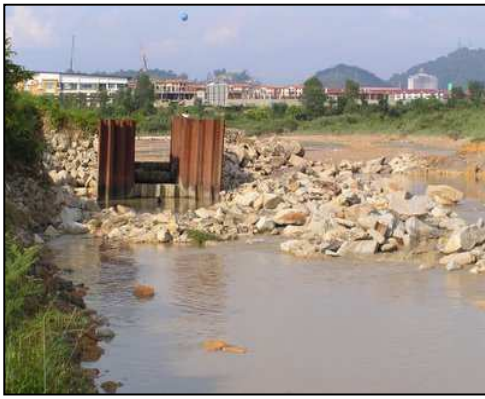
Fig.8: Broken bund on the site
