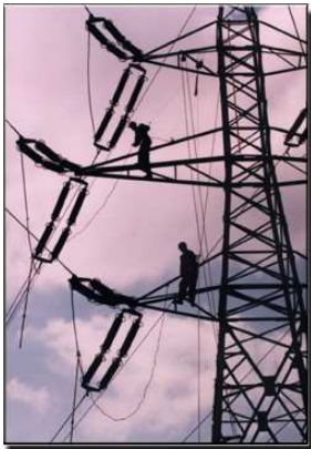
Fig. 4 – 400 kV line Cernavoda NPP
