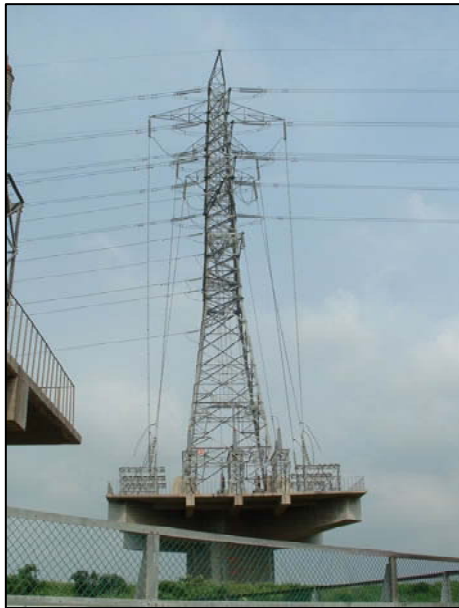
Fig.9 shows a cable connection station
