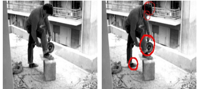
Figure 2A (left): Another random worksite activity. The student should comment on the appearance and the activity of the worker.
