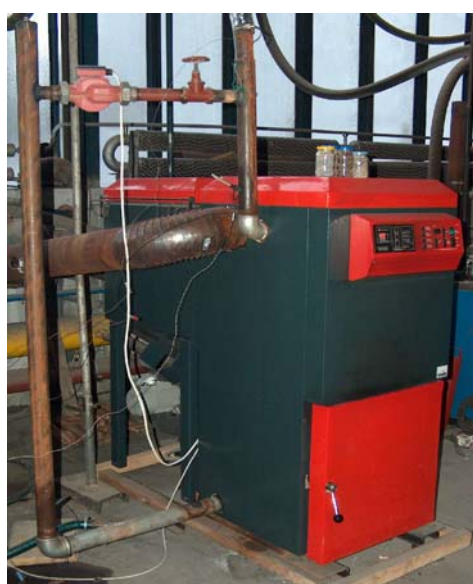
Fig. 1 The Verner A25 boiler – installation in the CTU labs
