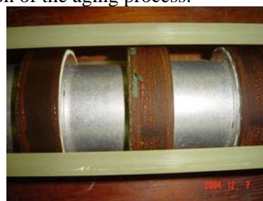
Fig. 4 – Varistors degraded by excessive heating.
