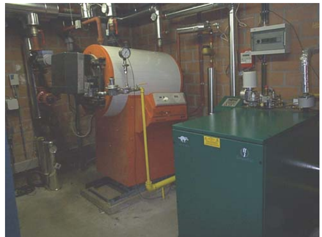
Fig. 3: Picture of the CHP integrated in the heating system
