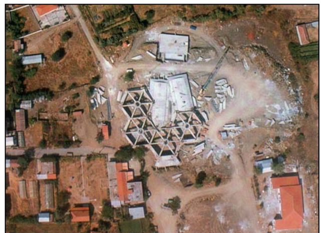
Fig. 8: Aerial view of the erection of the protective construction over the tombs' in Vergina
